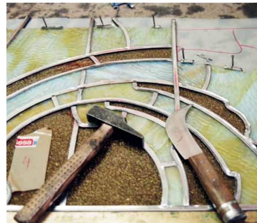
Detail of pieces from the main stairwell skylight during the restoration process
