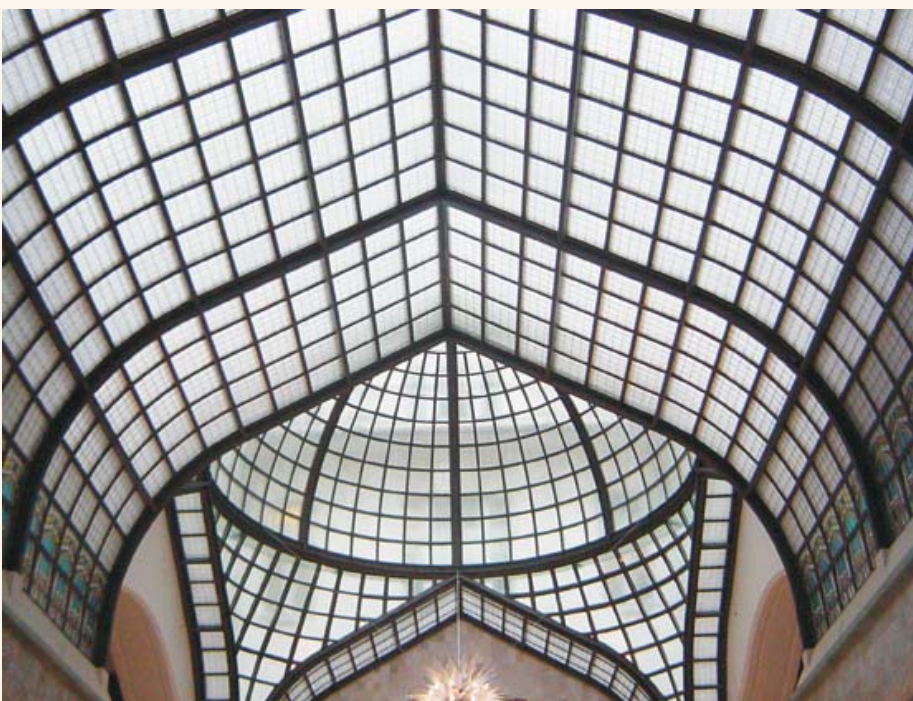
Stained glass roof structure of the foyer Estructura de la coberta de vitrall de la galeria
